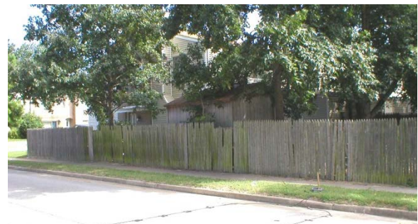
Deteriorating fences along roadway
